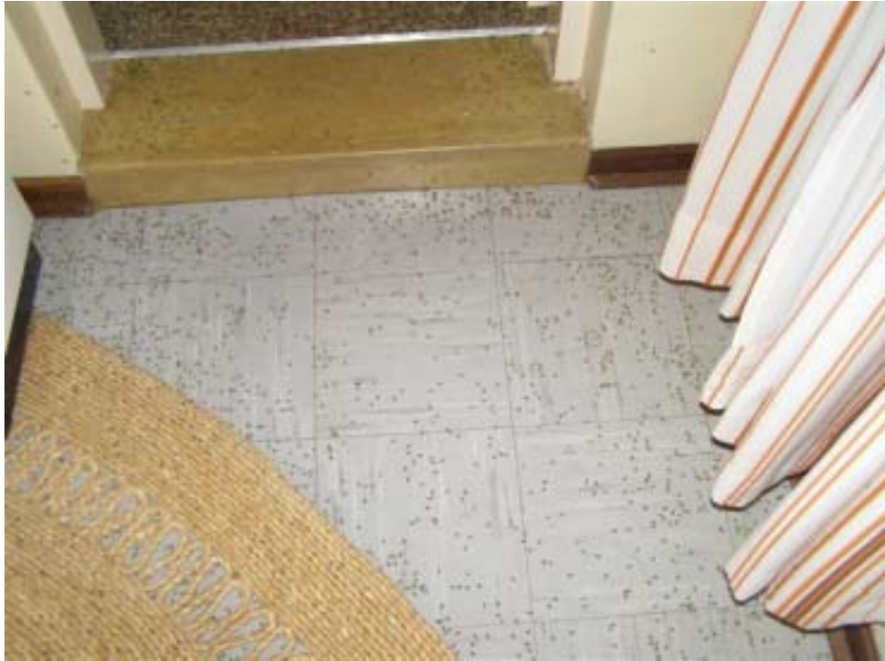
State of indoor floors every morning for more than three weeks
